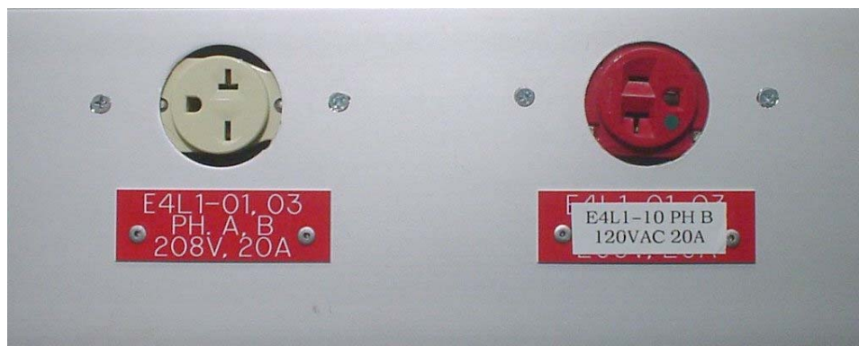
Figure 5 Emergency Generator Power Sockets
